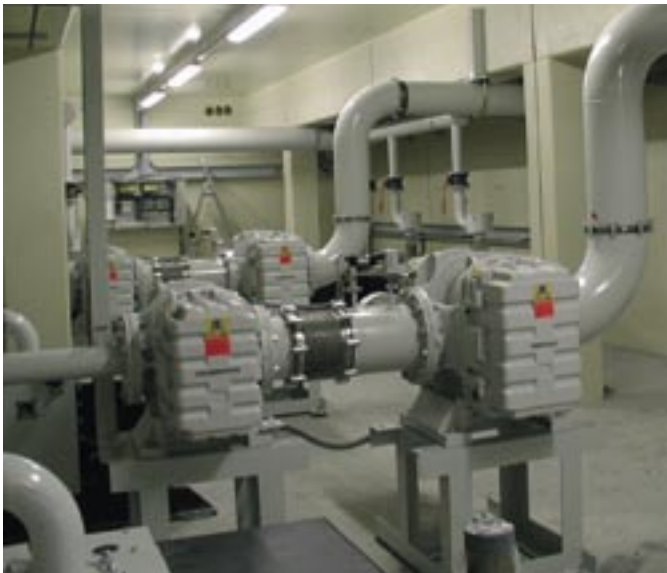
▼ 3-stage pumping set for 2 x 12.000 m 3 /h in coating technology ▼
