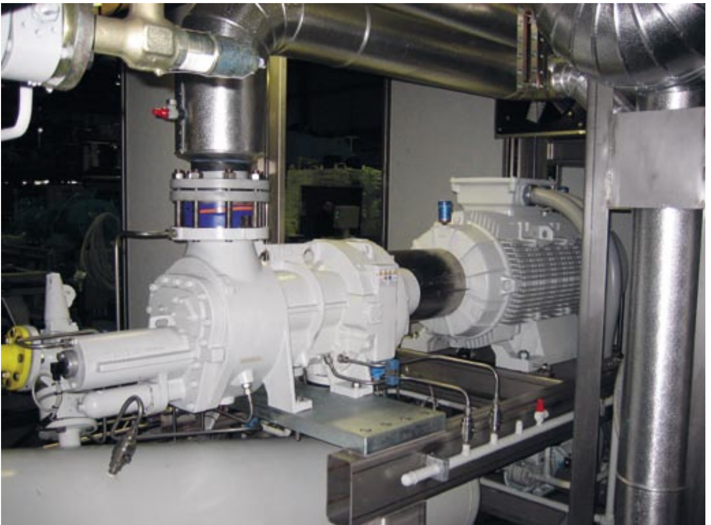
Picture 4: R717 2°C/+37°C / VMY 256 MHR driven via frequency converter
